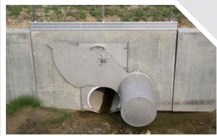
EQUIPEMENTS REGULATION HYDRAULIQUE
